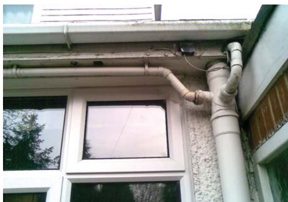
Example of exposed waste pipes
